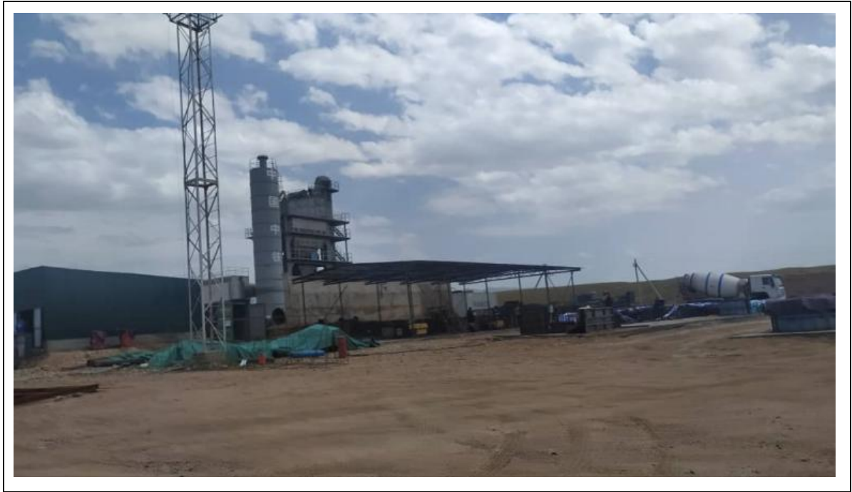
Figure 10 Asphalt plant at the production site.
